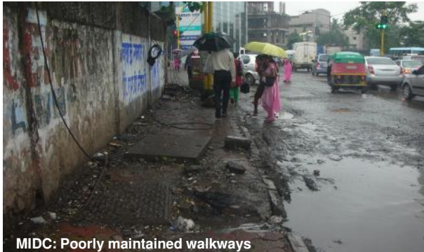
MIDC: Poorly maintained walkways
