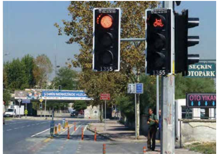
A bicycle signal is provided along a protected bicycle lane in Istanbul, Turkey (Source: © WRI)
